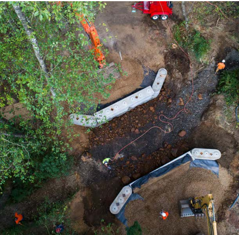
SSH worked with landowners to replace two barrier culverts with a bridge to open fish passage and restore the stream channel in Tomlinson Creek, a tributary of the Tillamook River and Tillamook Bay. Photo credit: Salmon SuperHWY.
